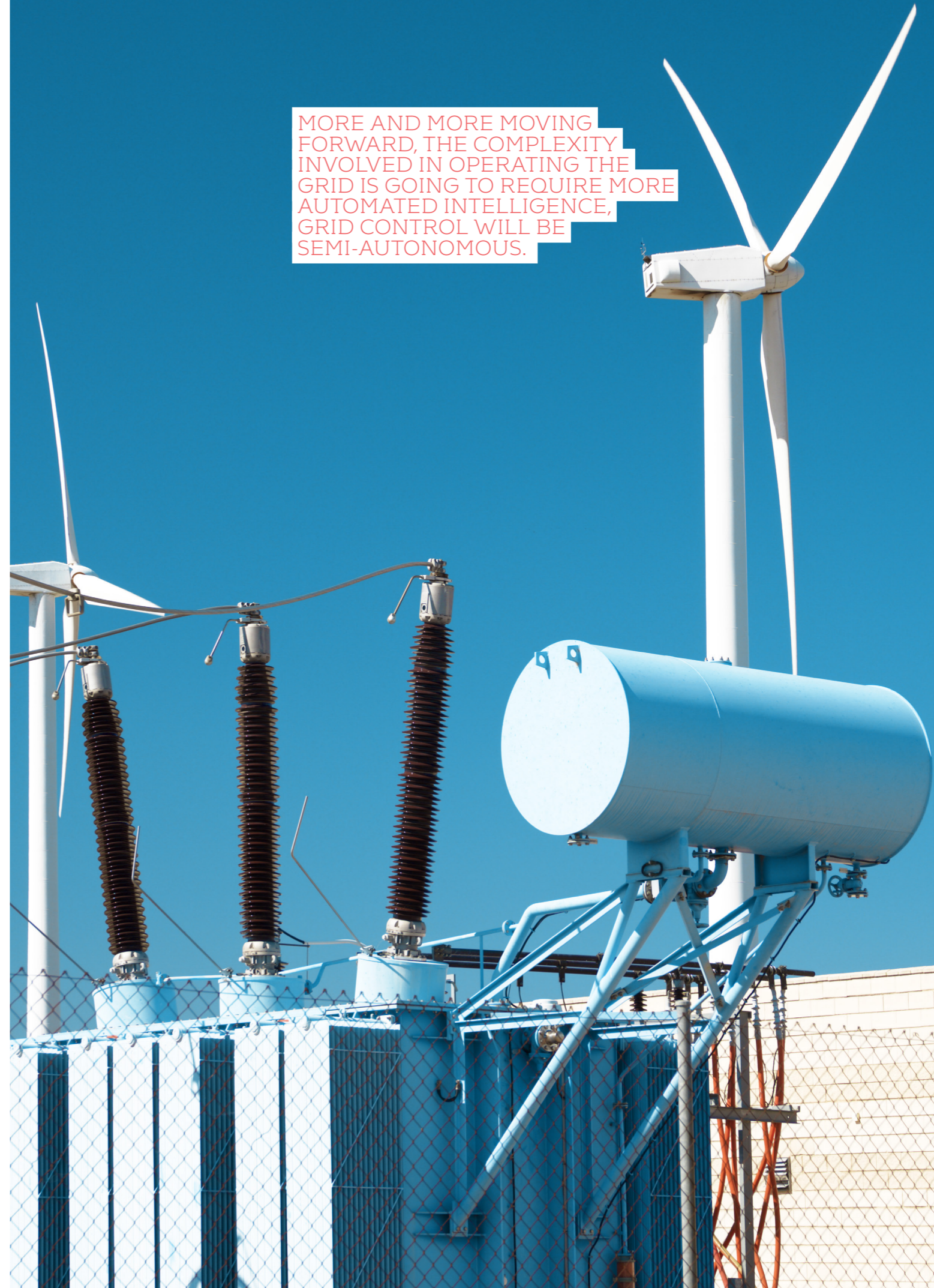
Photo: Camlin Energy
