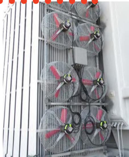
Figure 3b. Side mount fan tree configuration
