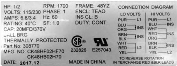
Figure 4. Existing fan nameplate to replace
