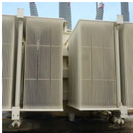
Before: Original manifold assemblies
