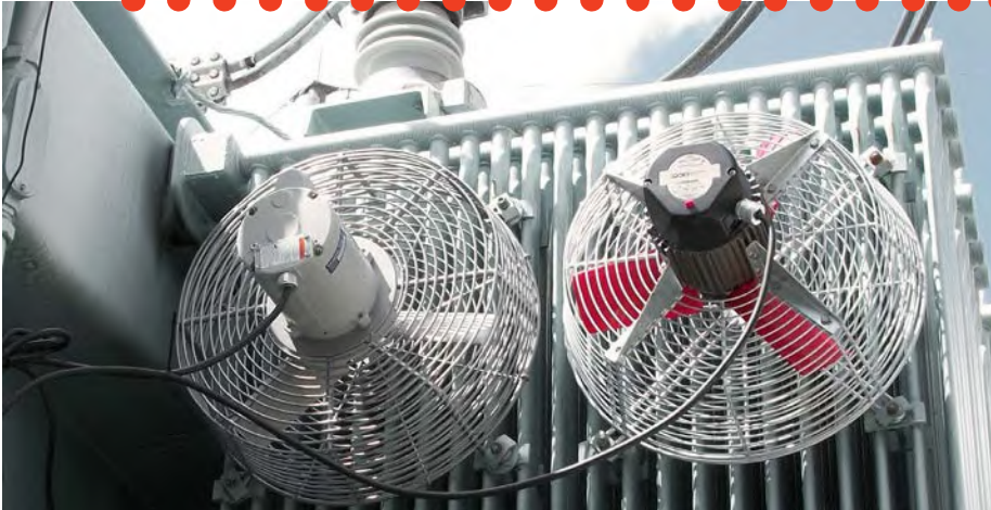
Figure 1. Old and new transformer cooling fan
