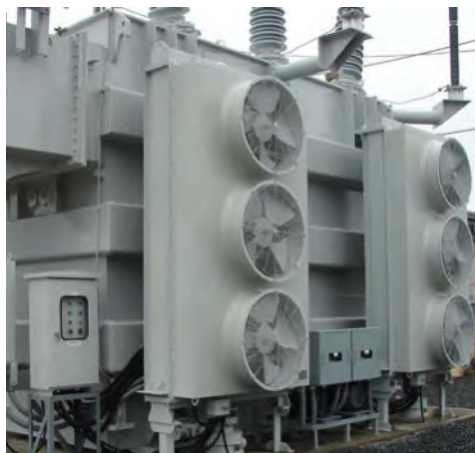
After: New fail-safe OFAF cooling system
