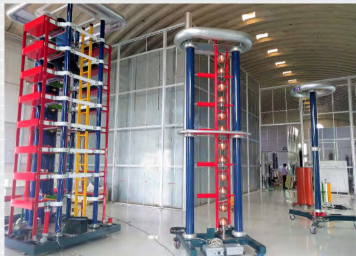
1500 kVp In-house impulse test lab
