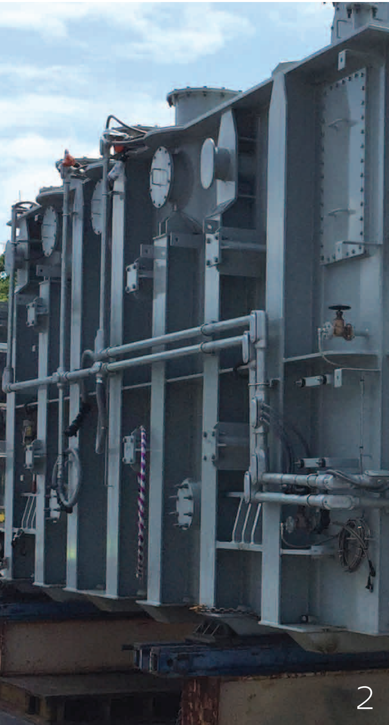
2) FirstEnergy's grid modernization program in Pennsylvania.
