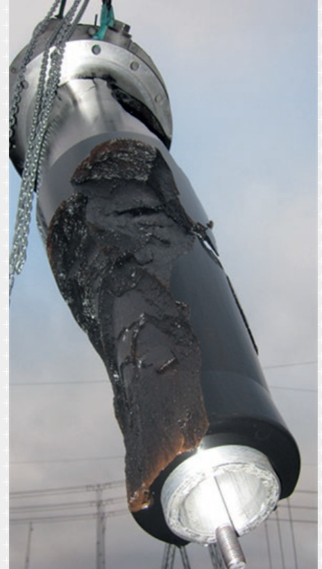
Figure 2 Picture of failed 400 kV RIP bushing installed on a shunt reactor with high impedance to earth and exposed to VFT.
