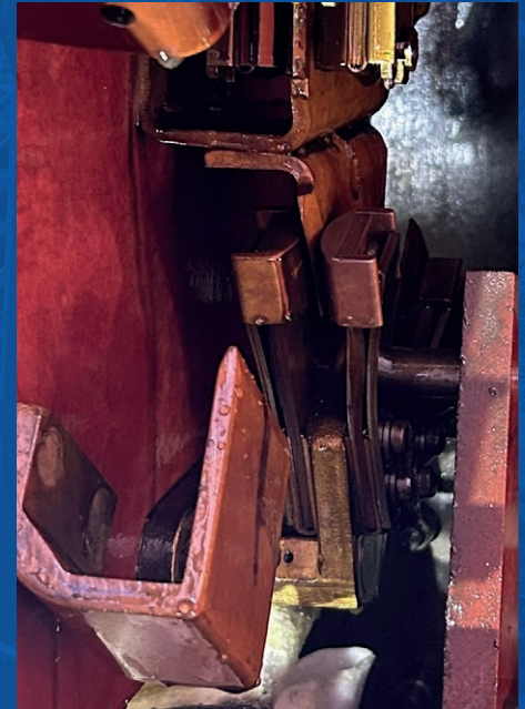
Poor Surface Contact
