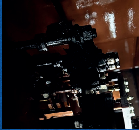
Figure 1: Burnt Reversing Switch from Outside Phase
