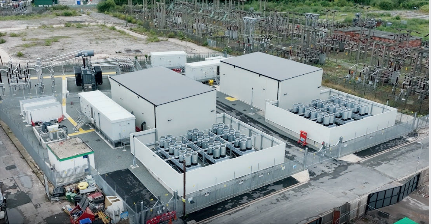
Figure 3 – Lister Drive is the world’s first application of ABB’s high-inertia SC configuration – housed in the two gray buildings.
