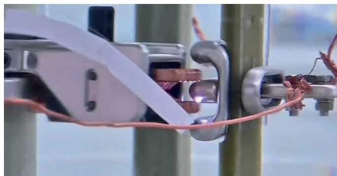
Figure 7: Discharge phenomenon when the tap changer performs a change-over switching in reverse phase between the contact bars
