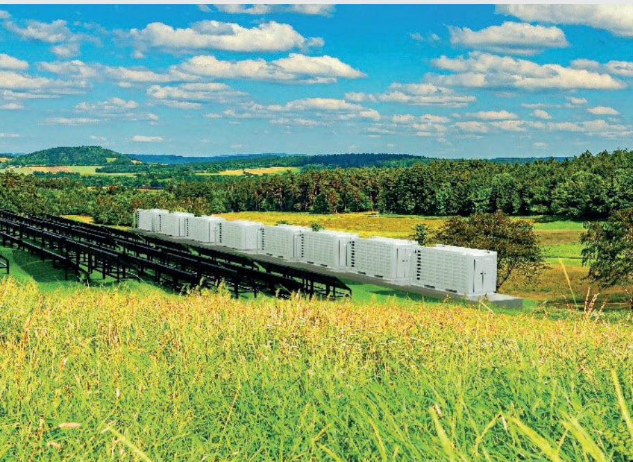
Figure 4 – Typical BESS installation supporting a solar farm
