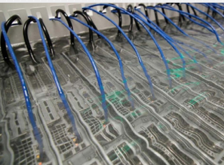
Computer processing equipment submerged with immersion cooling fluid
