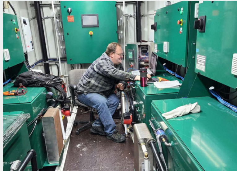
An employee with Mindful Energy Solutions, Inc. monitors tailored immersion cooling systems at an agricultural customer site
