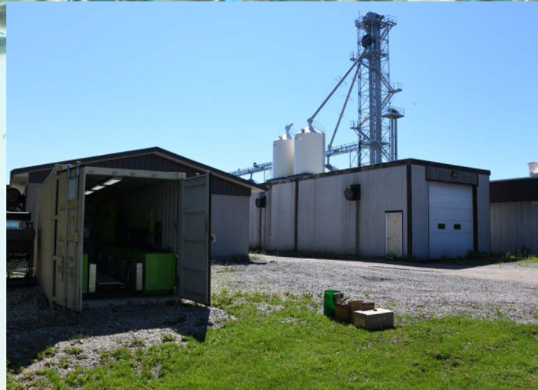
Data mining immersion cooling tanks positioned at a large ag operation in Manitoba provides an affordable, renewable heating source for their operations
