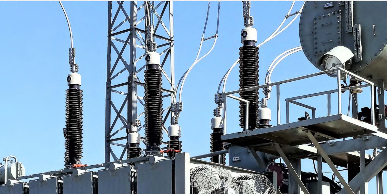
YASH MAKE 145 KV OIP BUSHINGS RETEOFITTED ON A TRANSFORMER TO REPLACE OLD SRBP BUSHINGS
