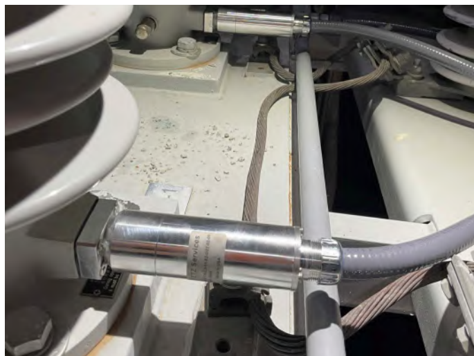
Figure 2. Bushing sensors installed on low-side bushings
