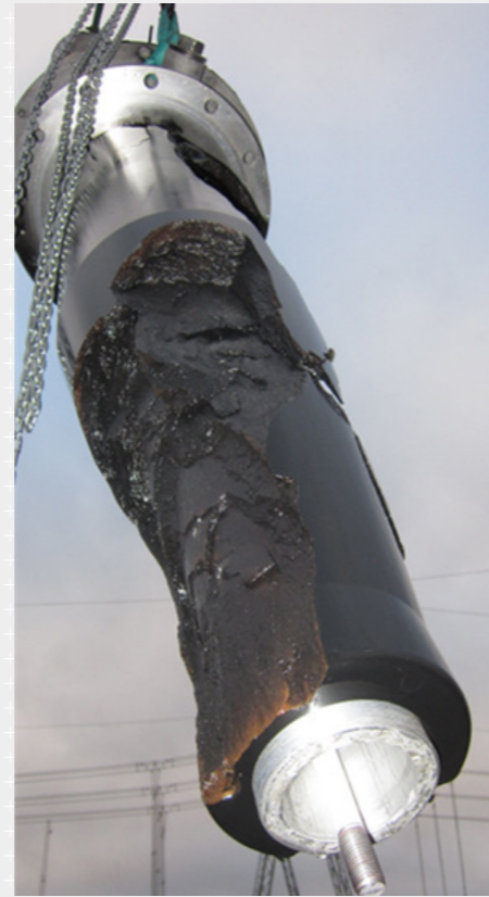
Figure 2 Picture of failed 400 kV RIP bushing installed on a shunt reactor with to high impedance to earth and exposed to VFT, and exposed to VFT.
