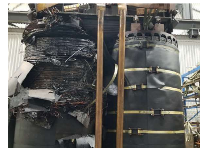
Figure 2. A Single Phase GSU with excessive moisture in the paper, and puncture from HV to LV through the barrier [4]
