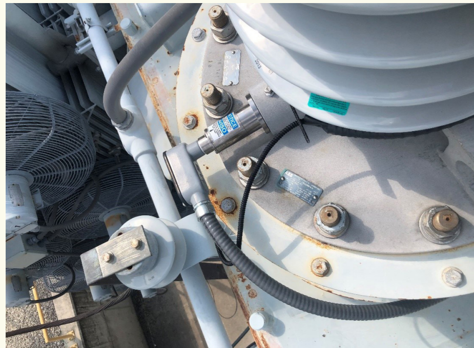
Figure 2: Bushing and Partial Discharge Sensor Installed on a GSU
