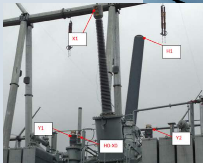
Figure 12: Picture showing the location of each bushing on single phase auto transformer with tertiary
