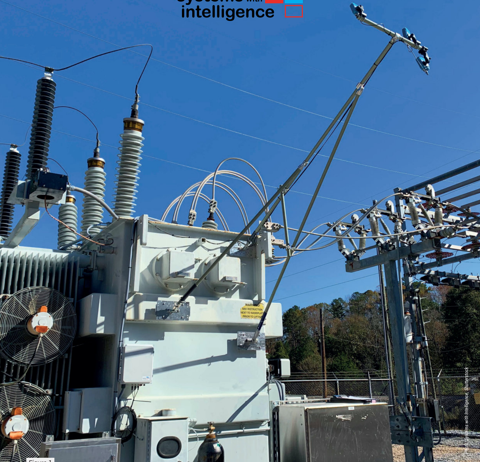
Figure 1 IM500 Quick Mount installed on Southern Company transformer.
