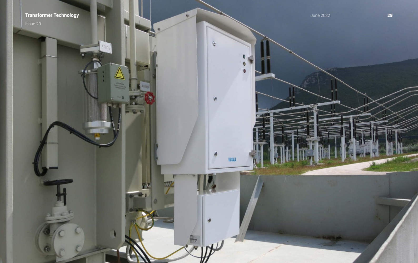
Online DGA monitor installed on a transformer (Photo courtesy of VAISALA)
