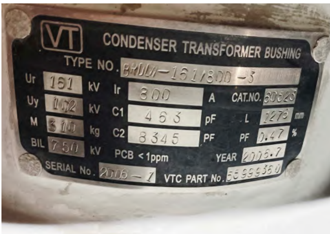
Figure 4. High-side bushing nameplate showing factory test data
