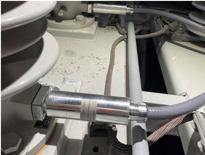
Figure 2. Bushing sensors installed on low-side bushings
