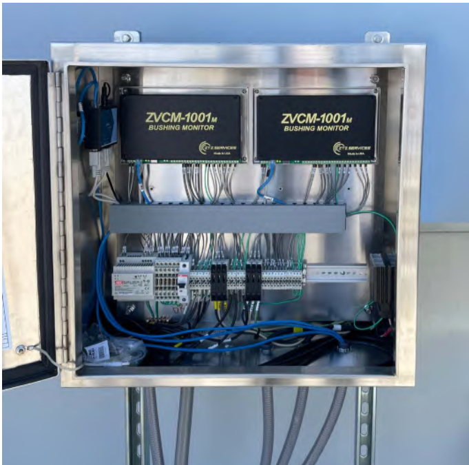
Figure 3. Two six-channel bushing monitors are installed beside the transformer
