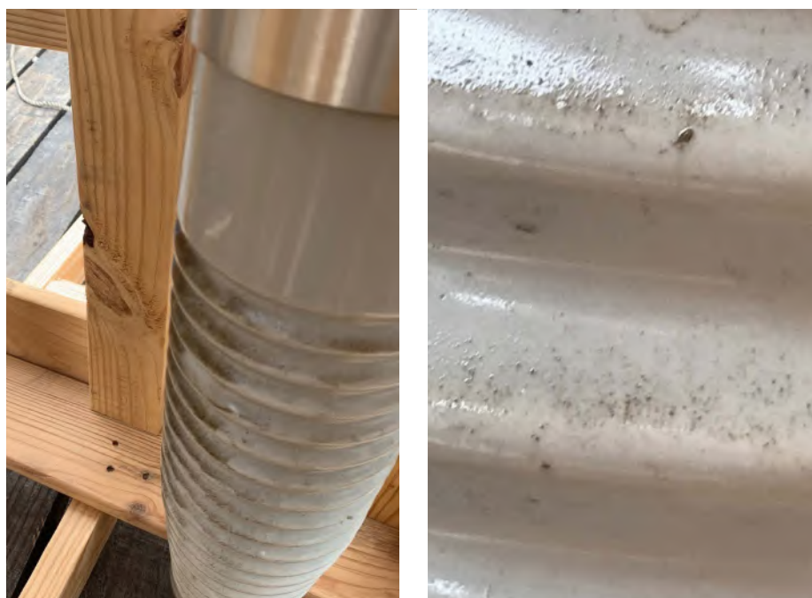
Figure 2. HV bushing removed from the transformer – surface contamination
