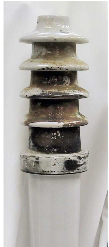
Figure 1. Hot oil and fire soot deposits
