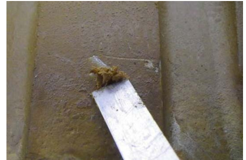
Figure 4. Sludge found in bushing head
