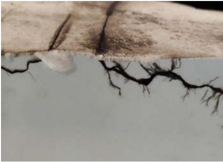
Figure 6. Arc tracking on internal porcelain
