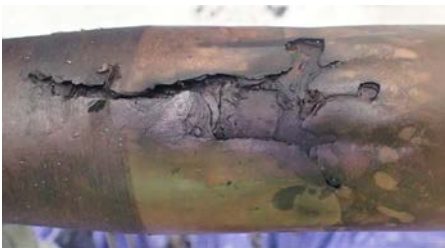
Figure 8. Arcing through core
