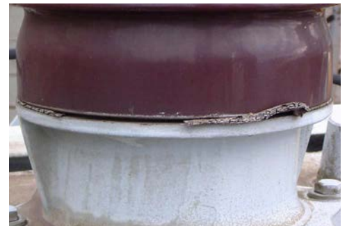
Figure 2. Compromised bushing gasket at flange-upper porcelain interface
