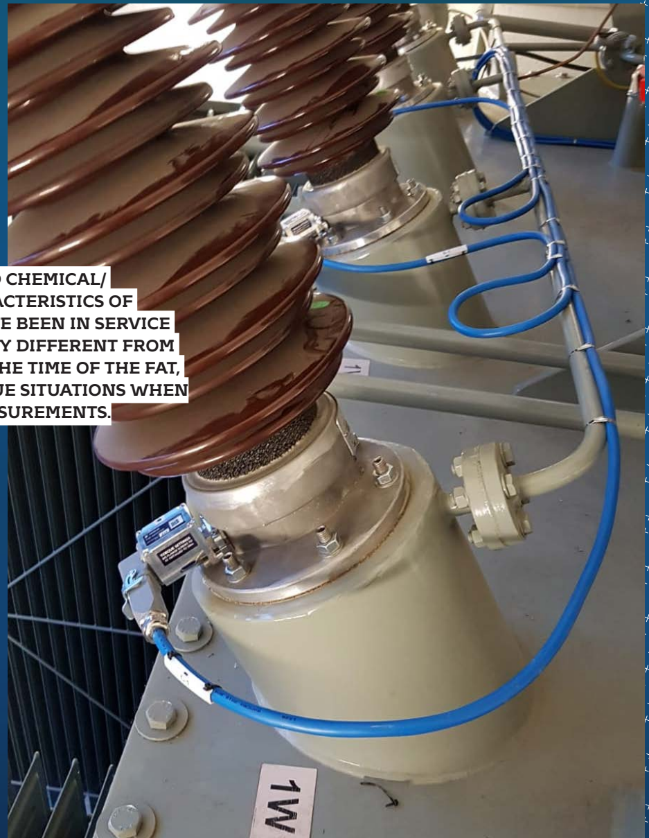
Figure 1. Bushing adaptor installed at the test tap for PD and Leakage Current online monitoring.
