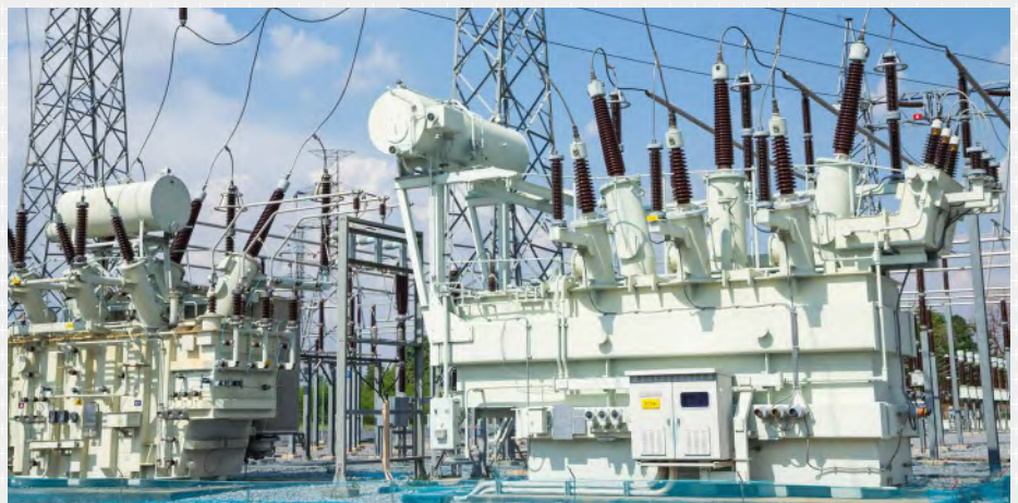
Figure 2. The complexity of cooling transformers has increased over recent decades resulting in higher efficiency and less noise emissions.
