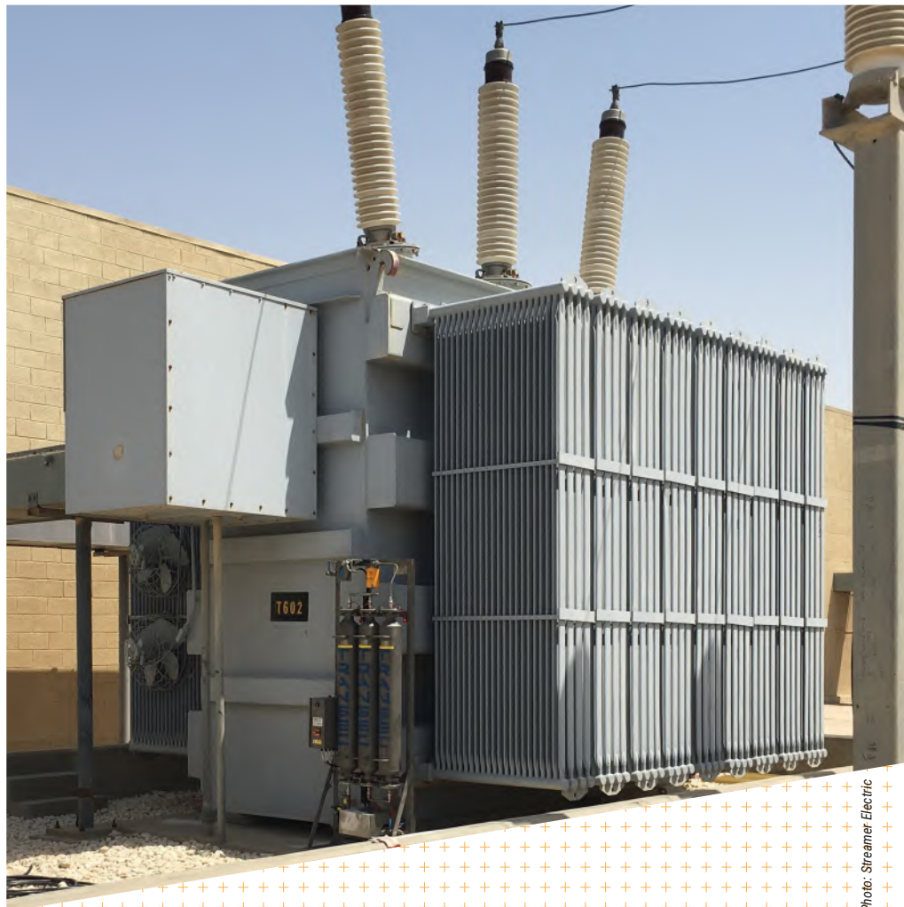
Figure 10. Online drying device with moisture monitoring installed on a transformer in Saudi Arabia's Abqaiq region
