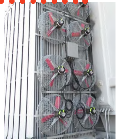
Figure 3b. Side mount fan tree configuration
