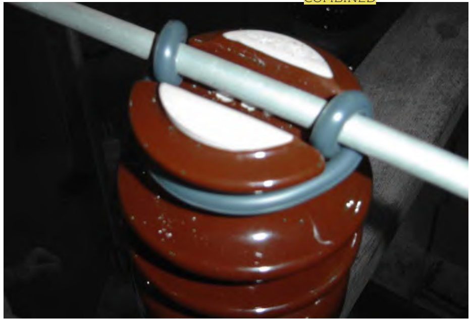
Figure 2. Tracking has begun to erode the enamel coating on this insulator. Moisture can impregnate and either super heat (arcing) or freeze. The insulative properties are failing and partial discharge will only worsen from here.
