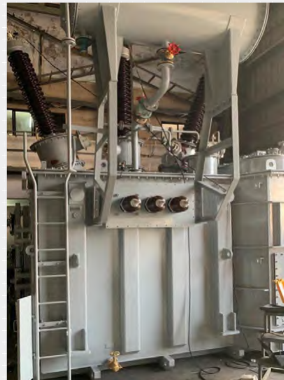
5,000/6,250 kVA FR3 oil immersed three-phase substation transformer
