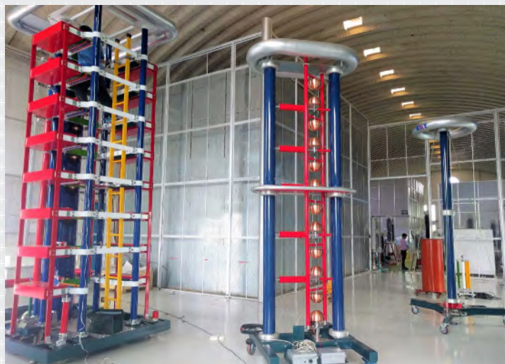
1500 kVp In-house impulse test lab
