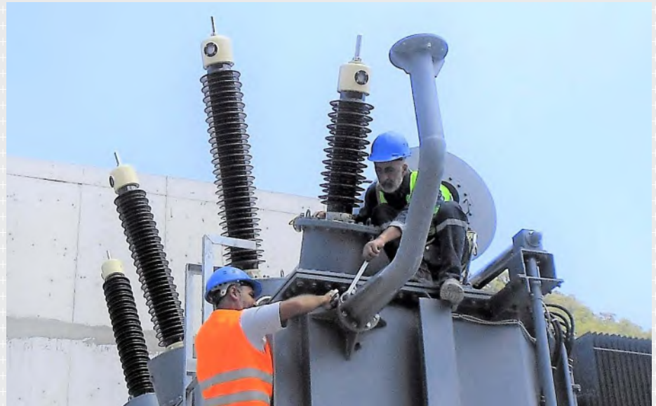
170 kV & 72.5 kV YASH OIP bushings. Transformer: Hyundai Heavy Industries. Site: Geothermal Power Plant – Turkey.
