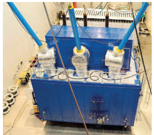
Figure 12. 400 kV transformers with MIDELE 7131 synthetic ester for Highbury substation in London, U.K. (Photo courtesy of Siemens Transformers)
