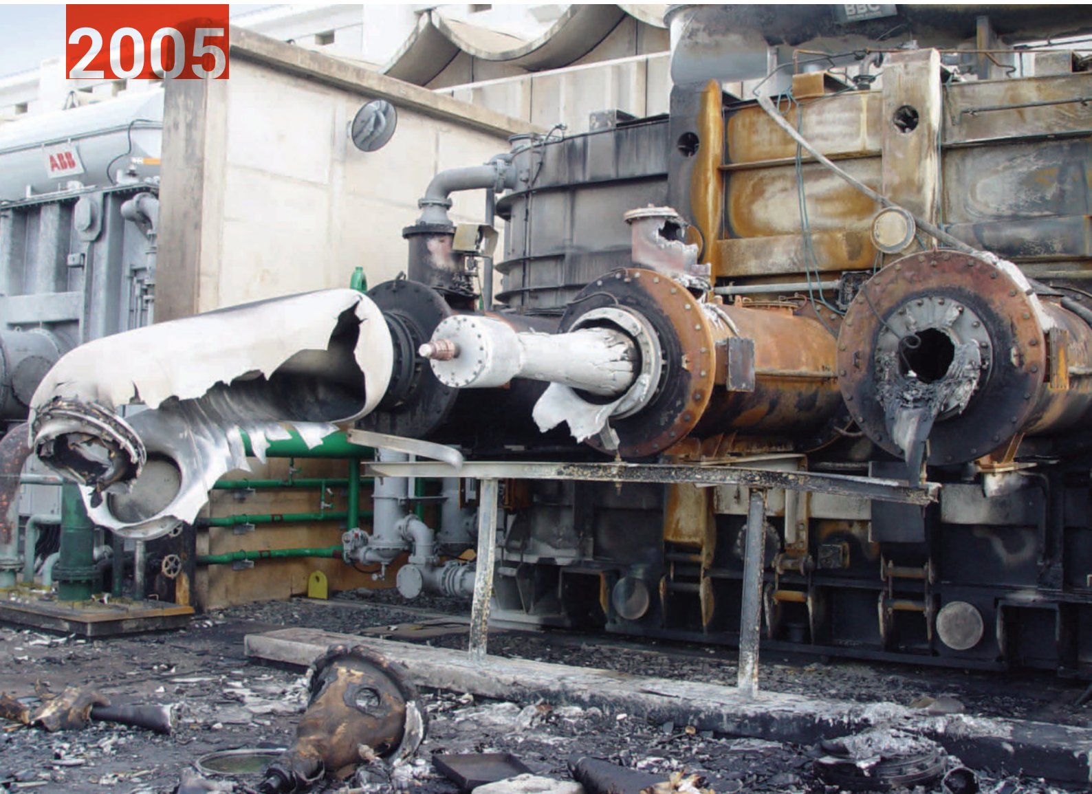
Figure 1. Catastrophic failures at the Tucuruí hydroelectric plant in 2005 (left) and 2007 (right)
