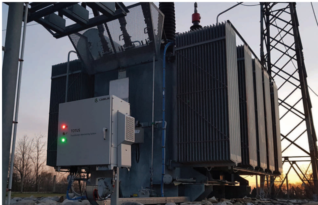
Figure 5. Online holistic monitoring system installed in 25 MVA GSU
