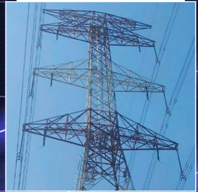
500kV Tower in South East Asia
