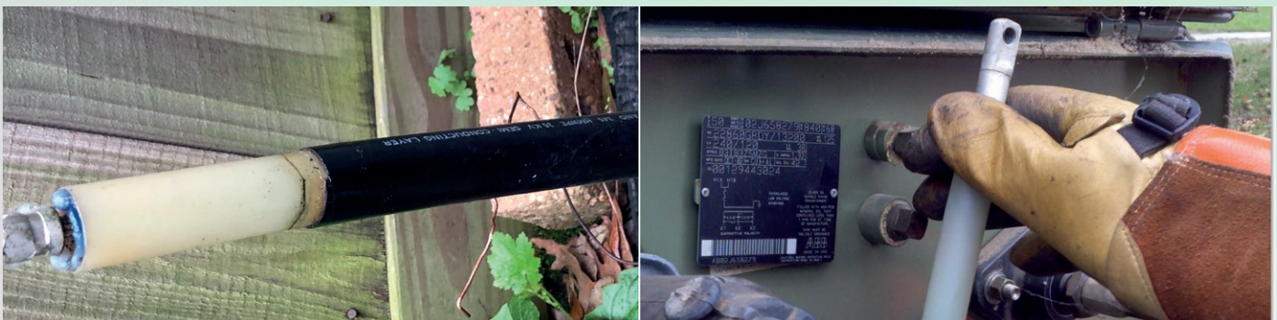
Example defects missed by a non-standardized PD test. Cable Defect (left), Splice defect (right)
