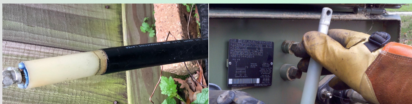
Example defects missed by a non-standardized PD test. Cable Defect (left), Splice defect (right)
