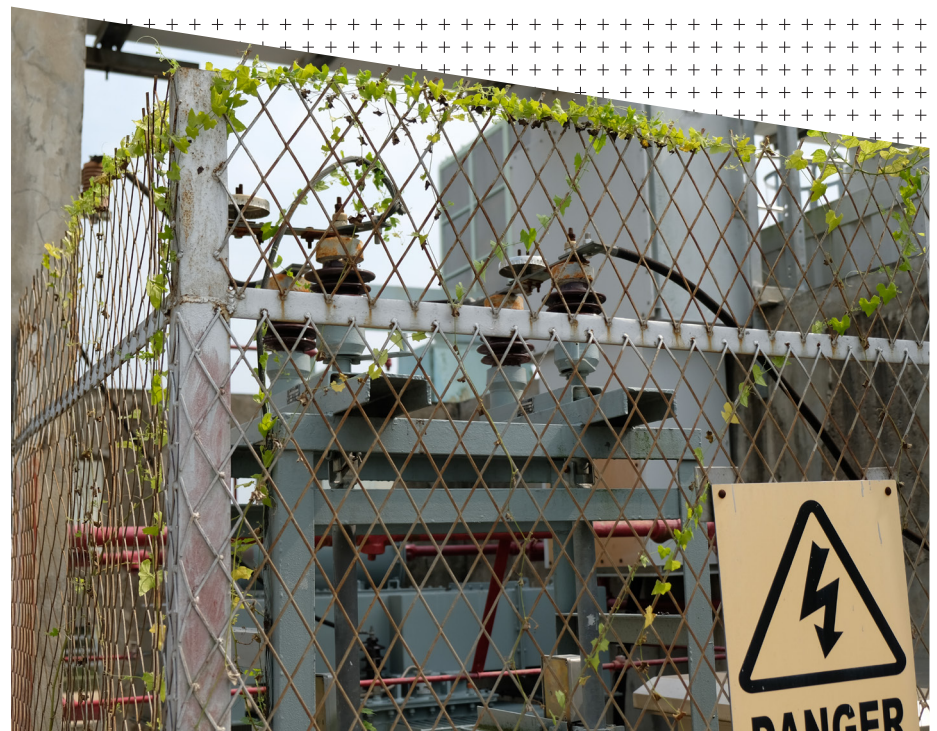
Figure 2. A traditional substation that requires easement, fencing and wildlife protection
