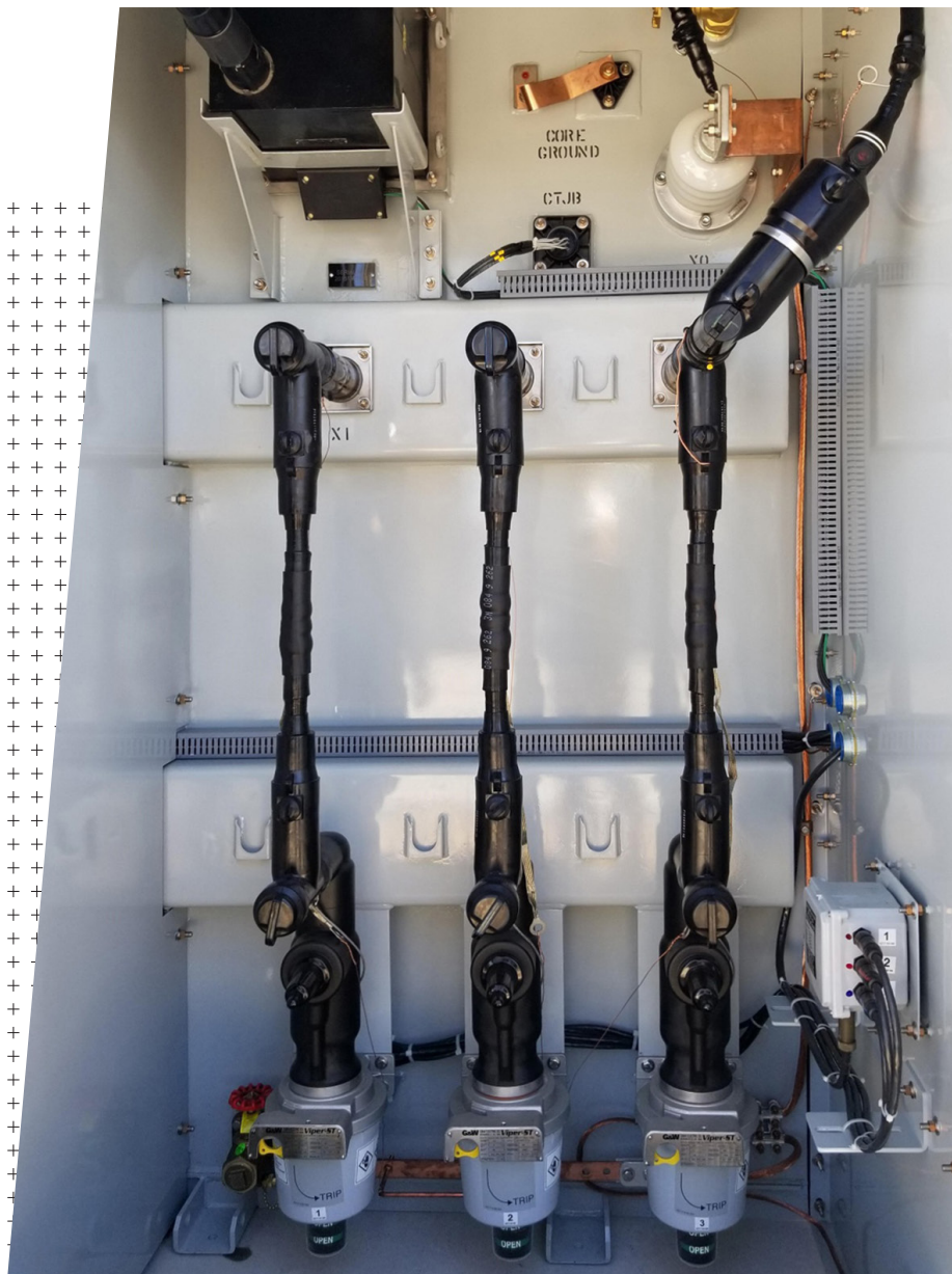
Figure 5. Cable connections are dead-front inside the pad-mounted transformer
