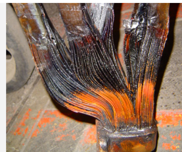
Figure 6: Overheated brazed connections at the bottom end of the LV winding lead.
